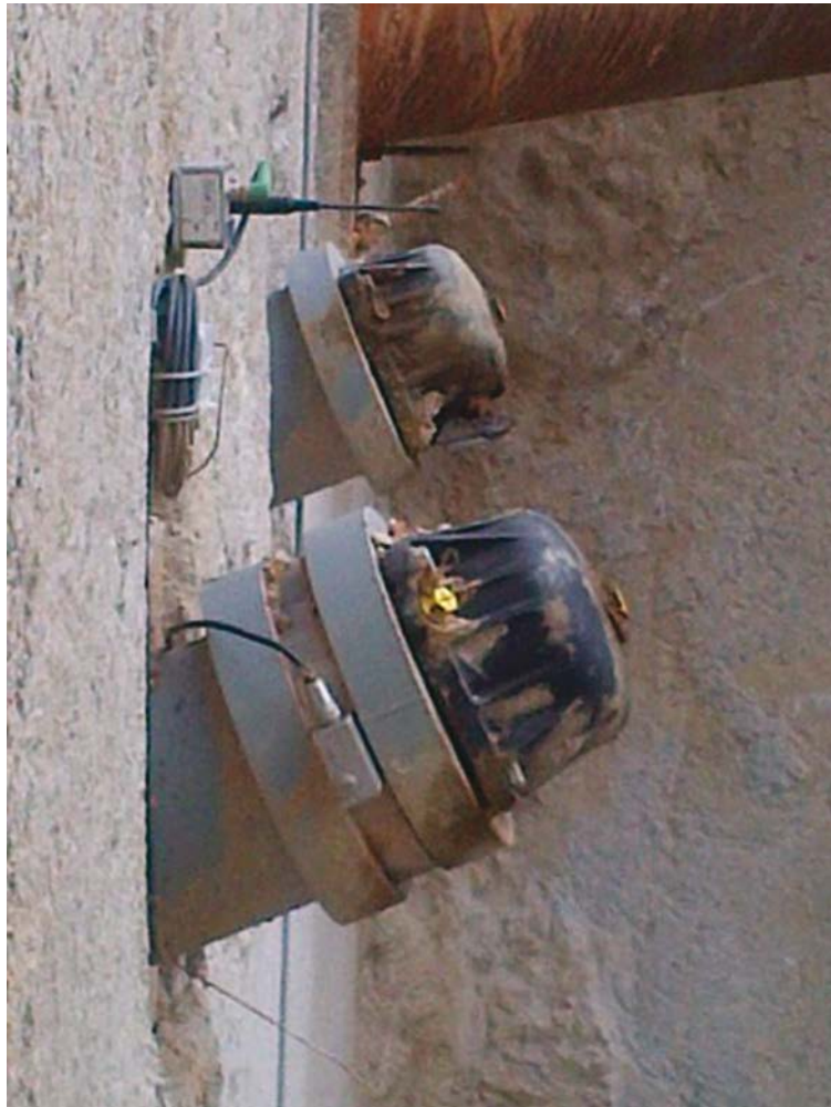
Picture 8.6: instrumented anchor head with radio signal (at the forefront) (© Freyssinet)
