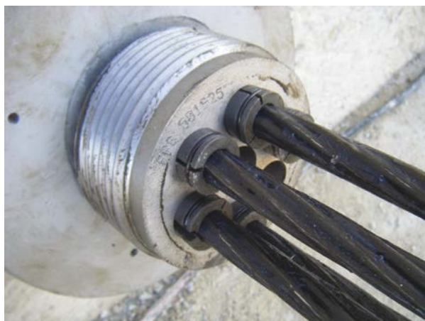
Picture 7.19b: Installation of the anchoring block and wedges prior to stressing (© Soletanche Bachy)
