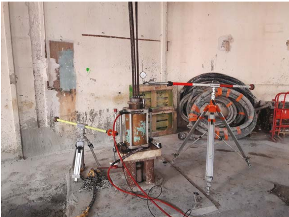
Picture I.5: Apparatus to measure displacements (© Spie Fondations)
