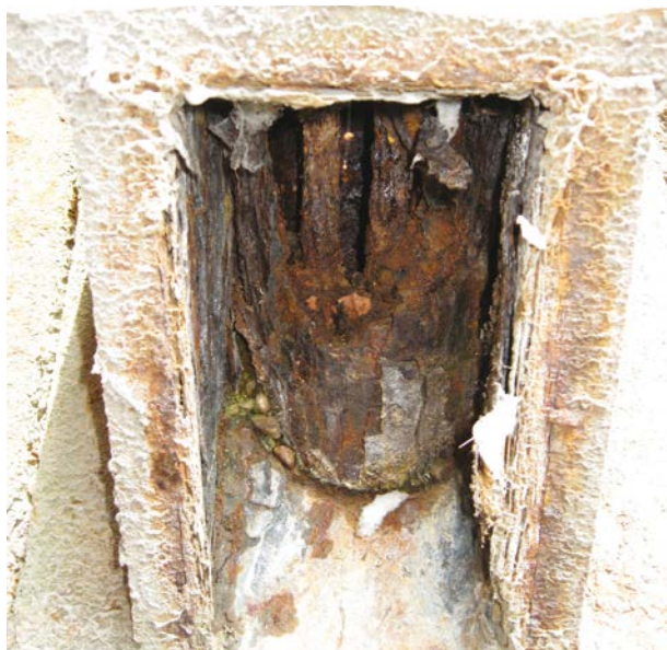
Picture 6.1: illustration of the effect of a protection defect at the anchor head level (©SMG)
