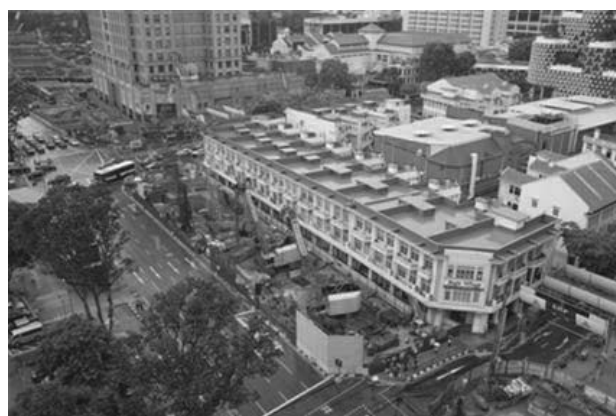
Figure 6. Excavation for the diaphragm walls in front of Bugis Village. Note the green ‘Ninja Turtle’ enclosure around the two excavation cranes.
