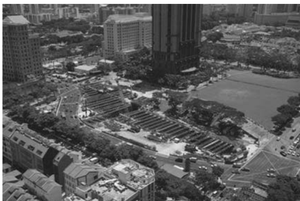
Figure 3. A view of the Station area showing the bottom up excavation and the Rochor Road diversion around the site.
