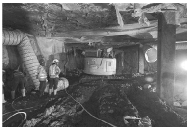
Figure 7. A view of the excavation in a ‘top down’ section, working below the roof slab.
