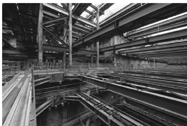
Figure 4. A picture from inside the Station showing the strutting required for the bottom up excavation.
