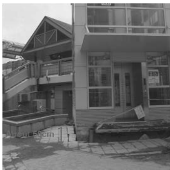
Figure 8. Large settlement induced at Shin-urayasu station
