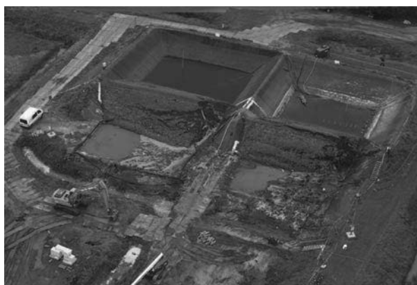
Figure 5. West and East dikes after failure.
