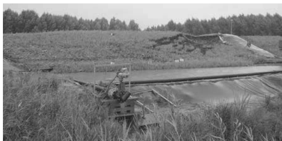
Figure 4. West dike close before failure.
