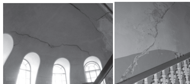
Fig. 6. Cracks in the vaults of the cathedral
