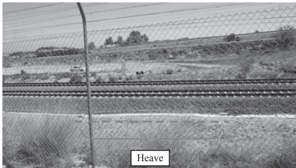
Figure 5. Bulge of the surface above the caisson. Observe the reduced thickness of the ballast layer
