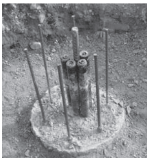
Figure 1. Typical pile heat exchanger at the site (after breaking down to pile cut off level).
