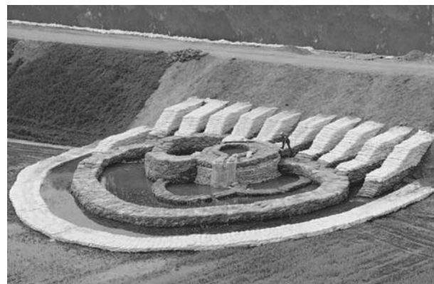
Figure 5. The giant piping at Tiszhasa/Hungary in 2000 and stabilizing measures (Nagy, 2011): Reduction of hydraulic gradient and lateral support of dyke slope.
