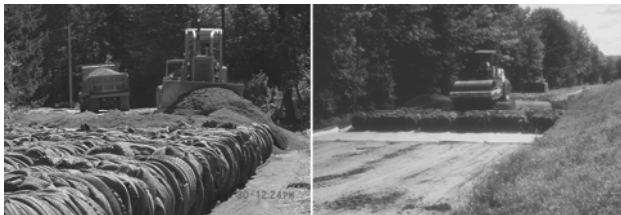
Figure 3. Bulldozing sand to fill voids, County Road 342 (CR342), 2000 (left); vibrating sand into inter-bale voids, CR647, 1999. (Courtesy Ken Smith, Chautauqua Co Dept of Public Facilities, NY.)
