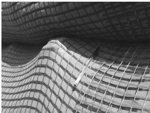
Figure 8. Uneven surface recorded at the wall #1 face.
