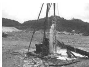
Figure 10. Ejection of leachate/gas
