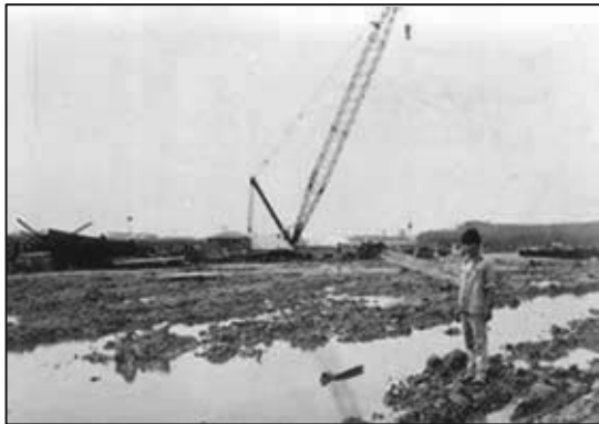
Figure 1. General condition of working platform without geogrids. (after Yong, Chan et al., 1990)
