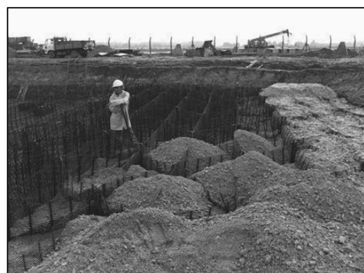
Figure 10. Install diaphragm with Tensor uniaxial geogrid and filling of geocells with granular materials.
