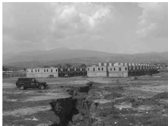
Figure 1. Crack in Chalco
