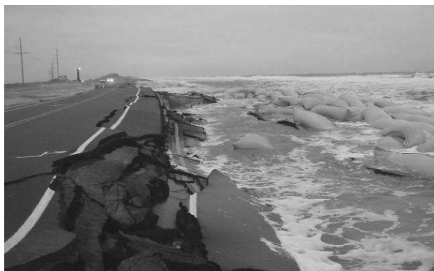
Figure 2. High ocean waves from Hurricane Sandy lap against Highway 12 and erode the underlying sand. (Photo: News & Observer, Nov. 14, 2012)
