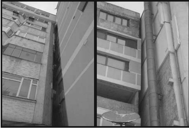
Figure 3. Photos showing on site displacements
