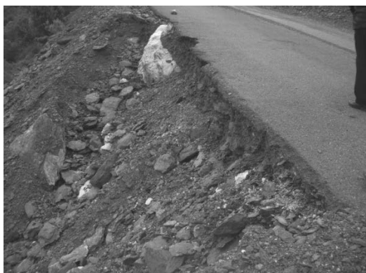
Figure 1. Photo of local slope failures
