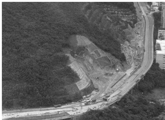
Figure 2: The Ching Cheung Road Landslide in 1997
