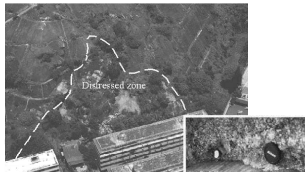
Figure 3: Laterally-persistent discontinuity infilled with slickensided kaolin and manganese oxide deposits at the 1999 Shek Kip Mei failure
