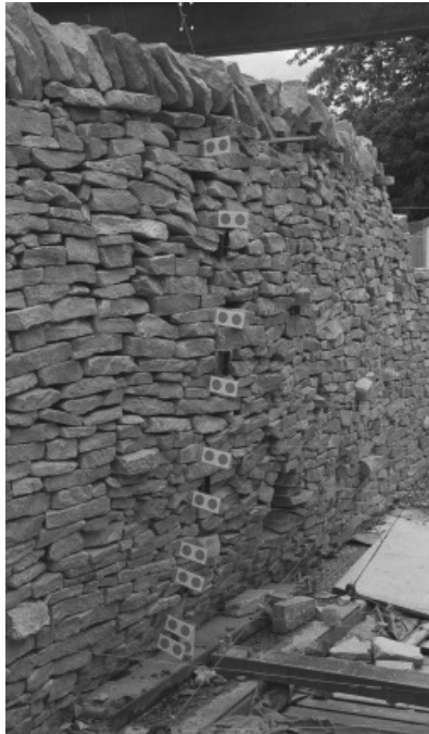
Figure 2. 2.4m high test wall at the University of Bath showing a classic bulged profile in a limestone wall of horizontal construction.
