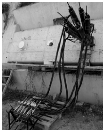
Figure 2. Test setup for simultaneous stressing of all strands of prestressed ground anchors using monostrand jacks.
