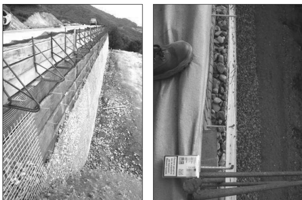
Figure 8. Left: construction stages (formwork, geogrids, anchor bars, facing), right: top view of the stone-filled facing used.
