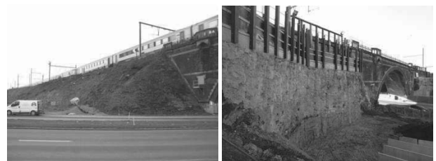
Figure 1. Picture of initial situation (left) and picture of the jet grout wall after excavation (right).
