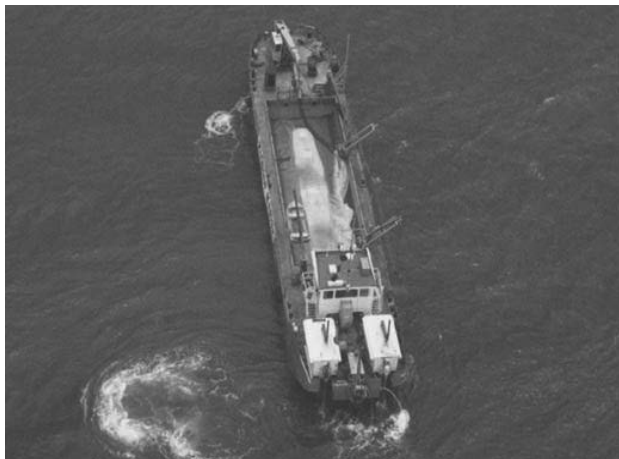
Figure 7. Hydraulic filling and placing of mega-sandcontainers with a split-bottom hopper dredger at Narrowneck Reef, Queensland, Australia (Heerten, 2010).
