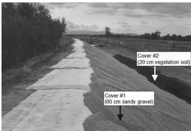
Figure 2. Dyke rehabilitation Kinzig 2000 / 2001 - Needle-punched GCL as water-side lining covered with locally available sandy gravel and top soil for gras vegetation.
