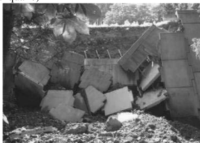
Photo 9. Collapse of facing panels in the sections where no fill substitution had taken place (After the 2011 Tohoku Earthquake)
