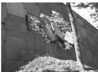
Photo 7. Collapse of facing panels by frost heaving of backfill. (Before 2008 the Iwate Miyagi Nairiku Earthquake)
