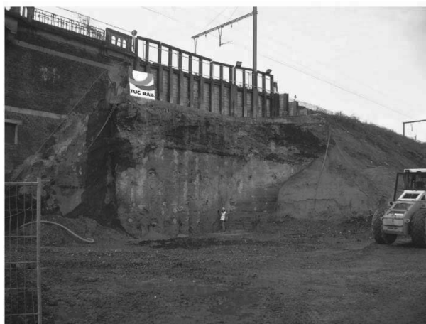
Figure 7. Photo of retaining wall after final excavation phase, after backfill for piling rig
