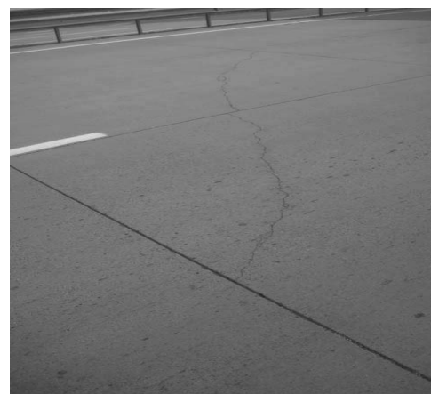
Figure 9. Oblique crack in cement concrete pavement of the highway “Astana-Burabai”
