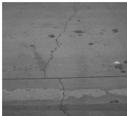
Figure 8. Transversal crack in cement concrete pavement of the highway “Astana-Burabai”
