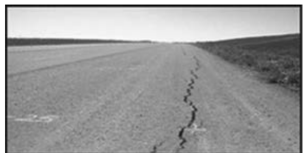
Figure 2. Longitudinal cracks near the edge of pavement
