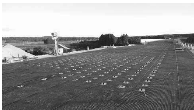
Photograph 3. Application of Confined-Reinforced Earth for actual highway embankment in Joban Highway, Fukushima, Japan, 2011.
