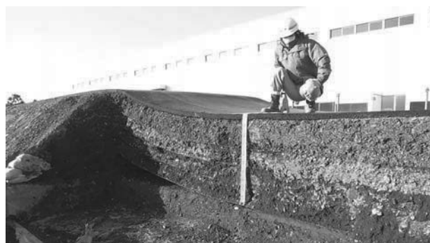
Photograph 7. Longitudinal cross section of Confined-Reinforced Earth and asphalt pavement after the Great East Japan Earthquake (550mm differential settlement).
