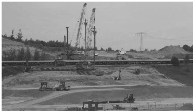
Figure 6. 15m high difference including ripping holes for the two devices RSV, CMC directly on BW2 and pressurimeter PMT in front.
