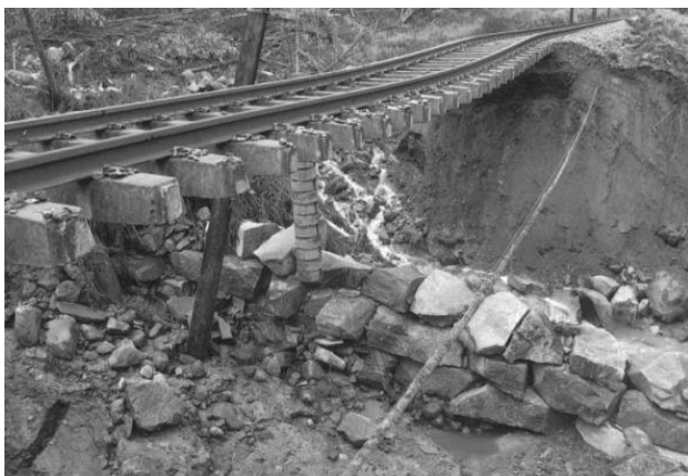
Figure 1. Example of total destruction of embankment around culvert near Ål, Bergensbanen railway line (Oslo to Bergen).
